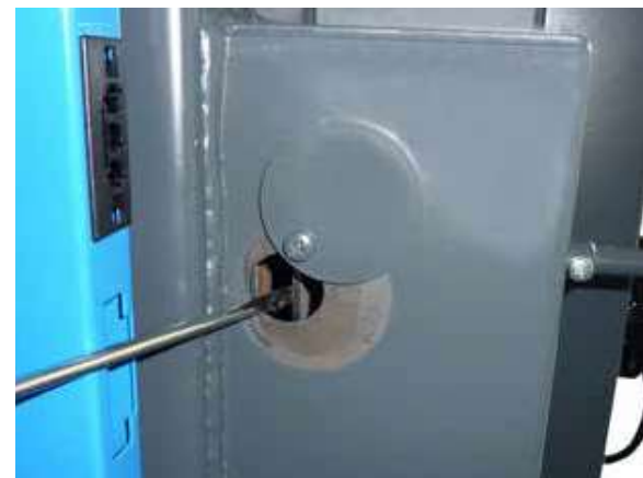
Checking and cleaning regulation of primary/secondary air ratio via cleaning lid
